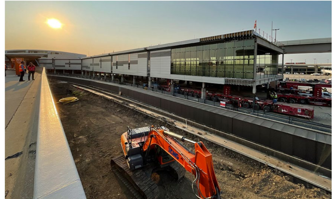
Six prefabricated sections of a new passenger concourse have been placed at DFW airport, a first for the domestic industry.
